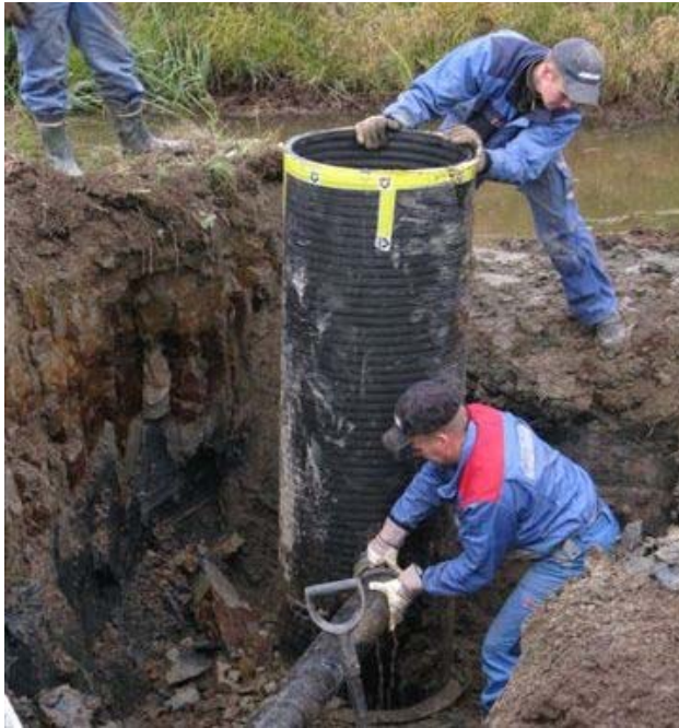
Installing a control well for regulated subsurface draining in an ASS landscape in Western Finland. Photo: Rainer Rosendahl
