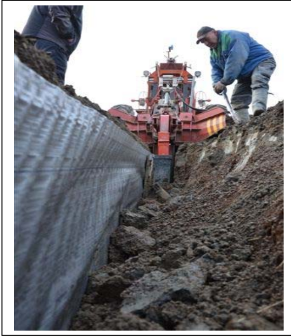
Installing a plastic wall to prevent flow of acid soil water in an ASS landscape in Western Finland. Photo: Rainer Rosendahl
