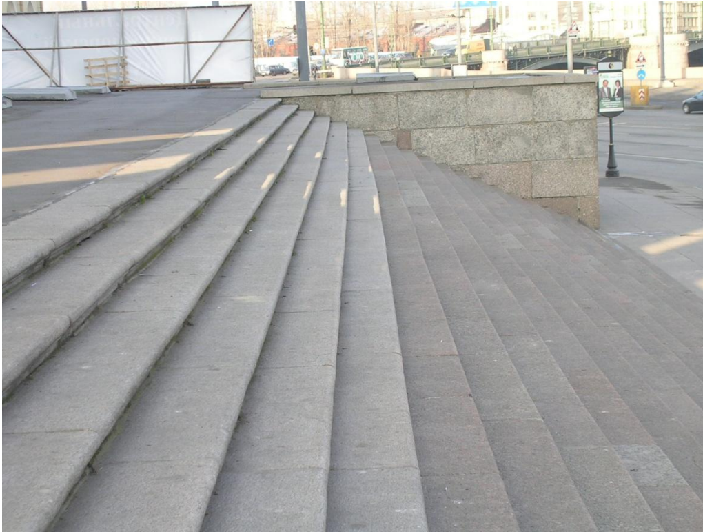
Figure 145 The granitic stairs of the stock exchange building have grey colours on the top part, and pink colour of the lower part..
